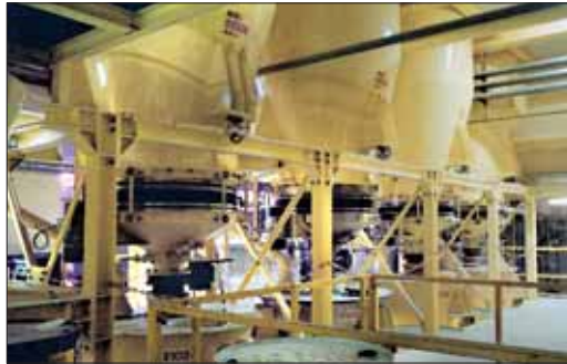
Figure 12: SX bin dischargers in a detergent factory
