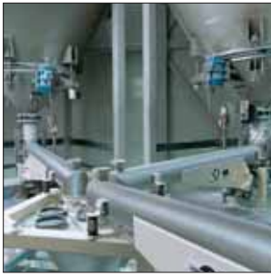
Figure 1: Vibrating tube conveyors feeding a weighing hopper
