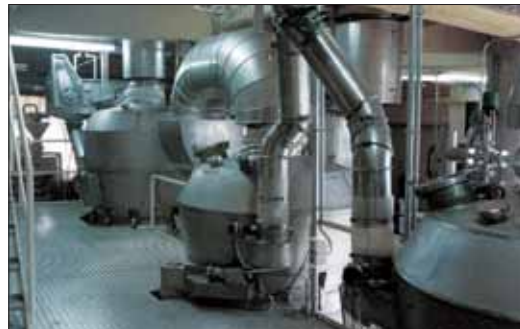
Figure 27: Vibratory fluid-bed batch dryer for roasting chopped almonds
