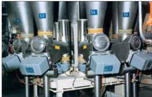
Figure 14: Bin discharging tube conveyors
